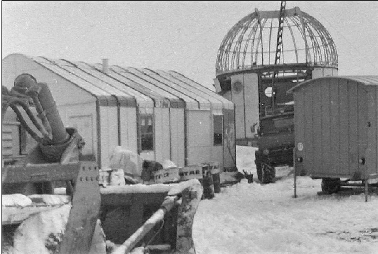
Figure 4: The house (left) and dome (right) under construction in the autumn of 1974 (courtesy: Paris Observatory).
